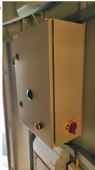
Fig. 1: Dome control box - red: main switch
