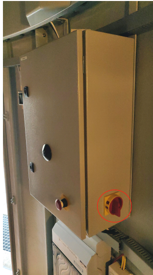
Fig. 1: Dome control box - red: main switch
