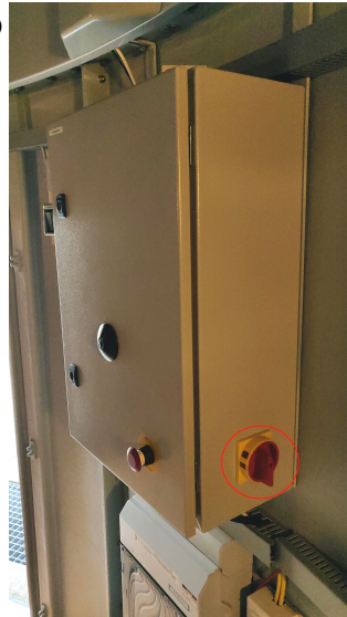
Fig. 1: Dome control box - red: main switch
