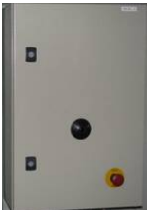
Control box with the emergency button
