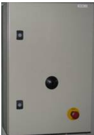
Control box with the emergency button
