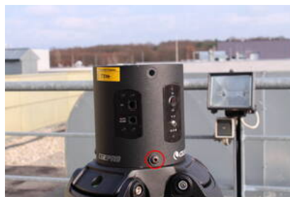
Fig. 2: Tripod with the electronic box (the red circle indicates one of the bolts that needs to be fastened)
