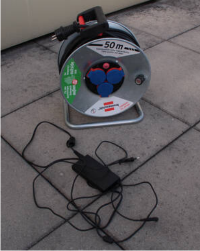
Fig. 10: mobile power supply and cable reel
